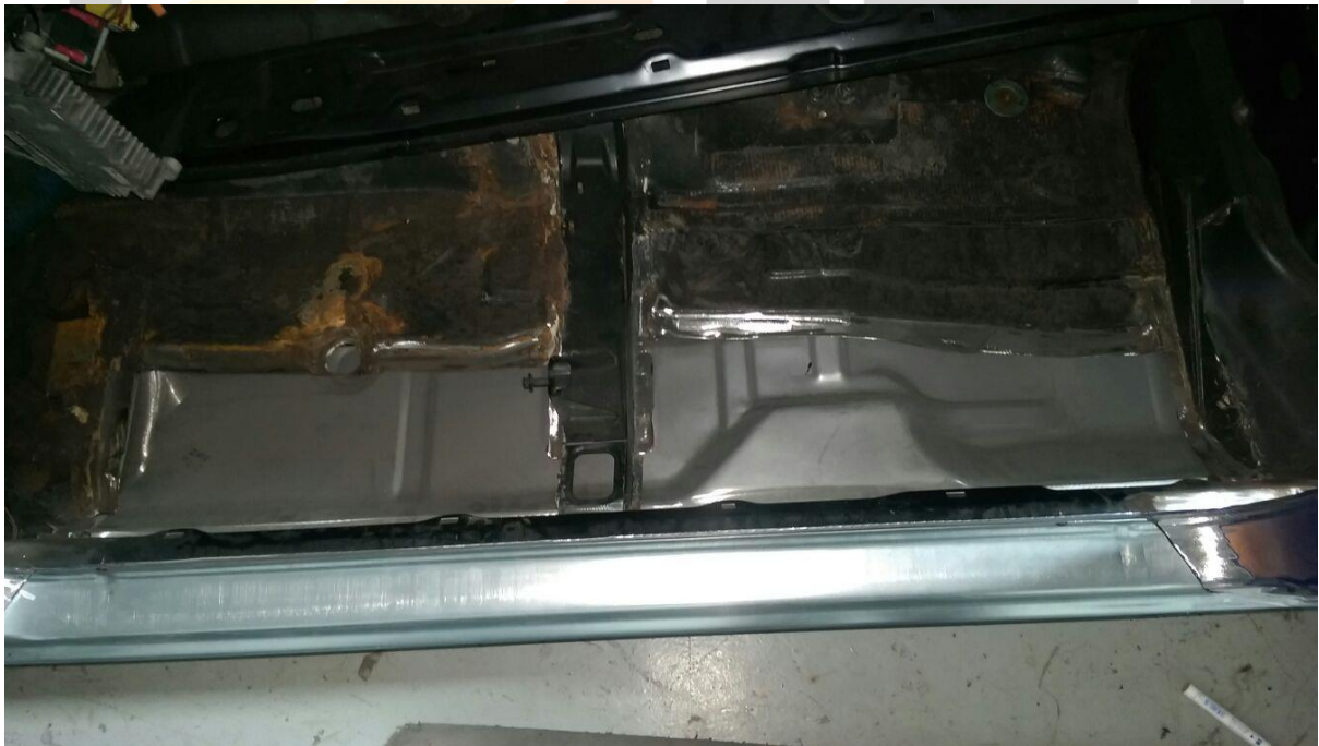
Old floor cut out and new one offered up for sizing and trimming
